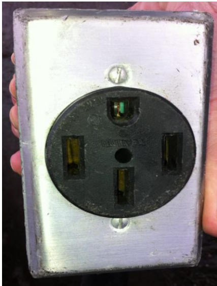
Outlet required at facility
